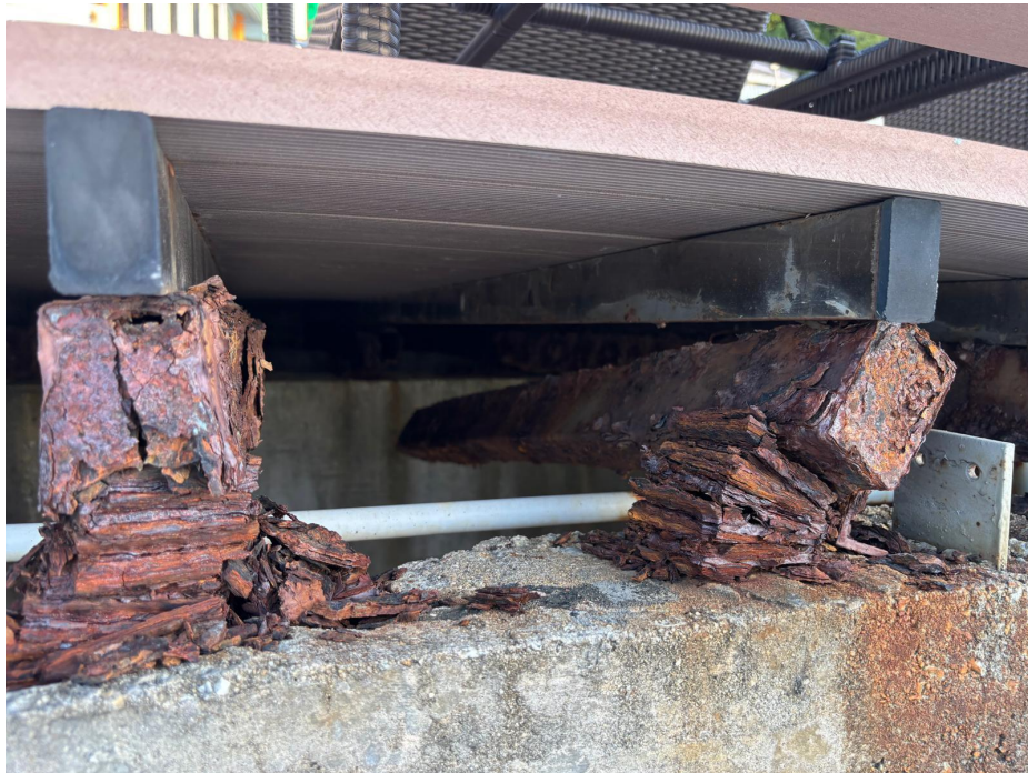
Figure 1: Current Condition of Timber Deck Steel Joist Onsite
